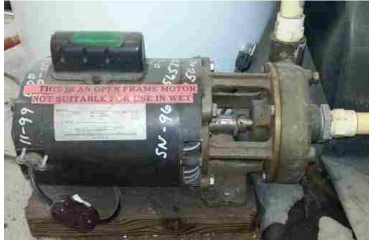
Figure 5.1. Pump used to circulate water in full scale curing system
