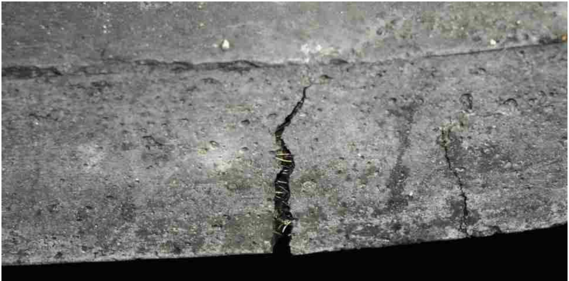
Figure 6.21. Panel B-3-2F-3.5 vertical crack on front edge after 2nd detonation
