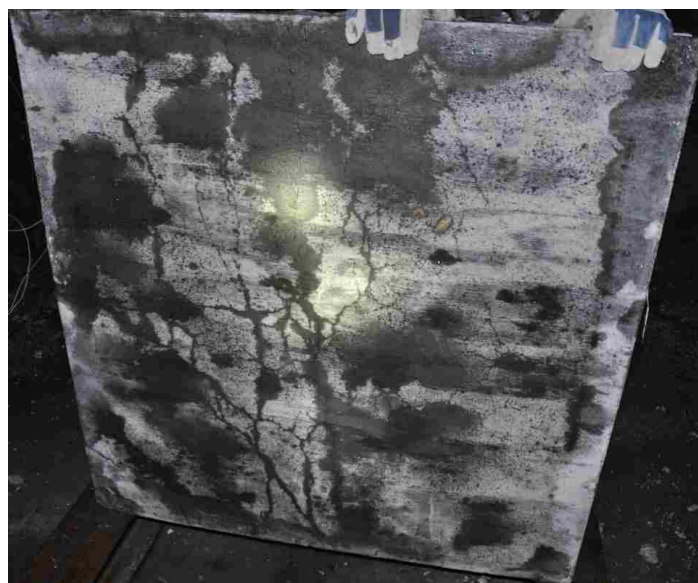
Figure 6.19. Bottom face of B-3-2F-3.5 after detonation
