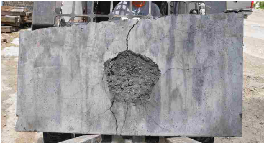
Figure 6.57. Back (tension) face of H-5-2F-3.5 after detonation
