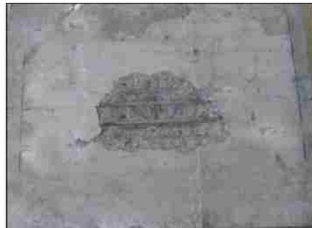
Panel 4 rear surface after explosion - Heavy scabbing, reinforcing bars exposed. - Cavity approximately 480 mm x 300 mm (18.9-in x 11.8-in), with a maximum depth of 50 mm (1.9-in) (1/2 section depth).
