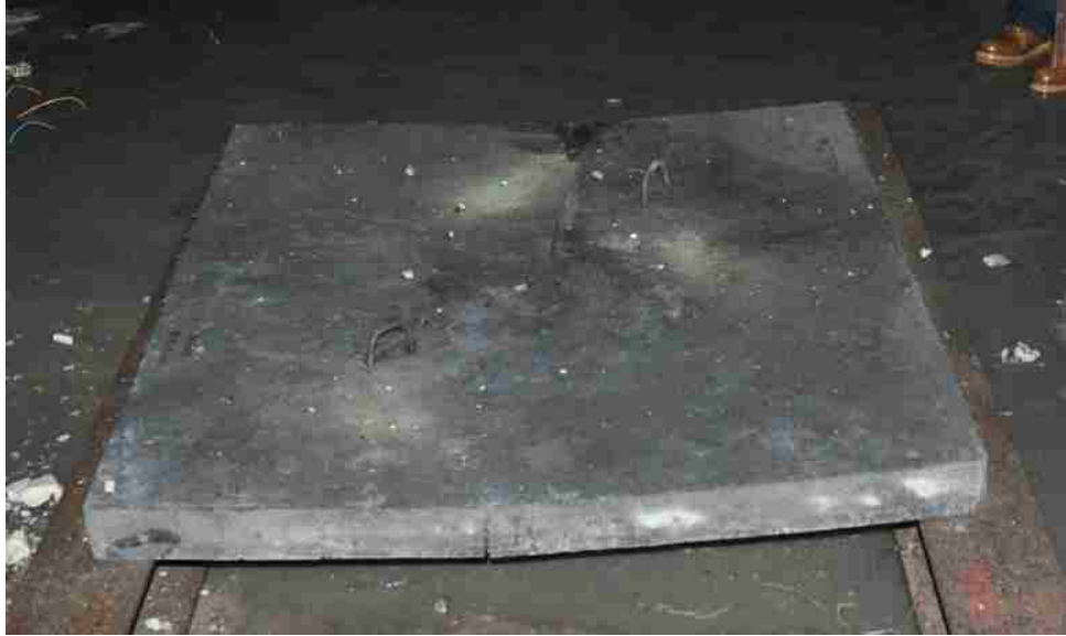
Figure 6.20. Panel B-3-2F-3.5 top face damage after 2nd detonation
