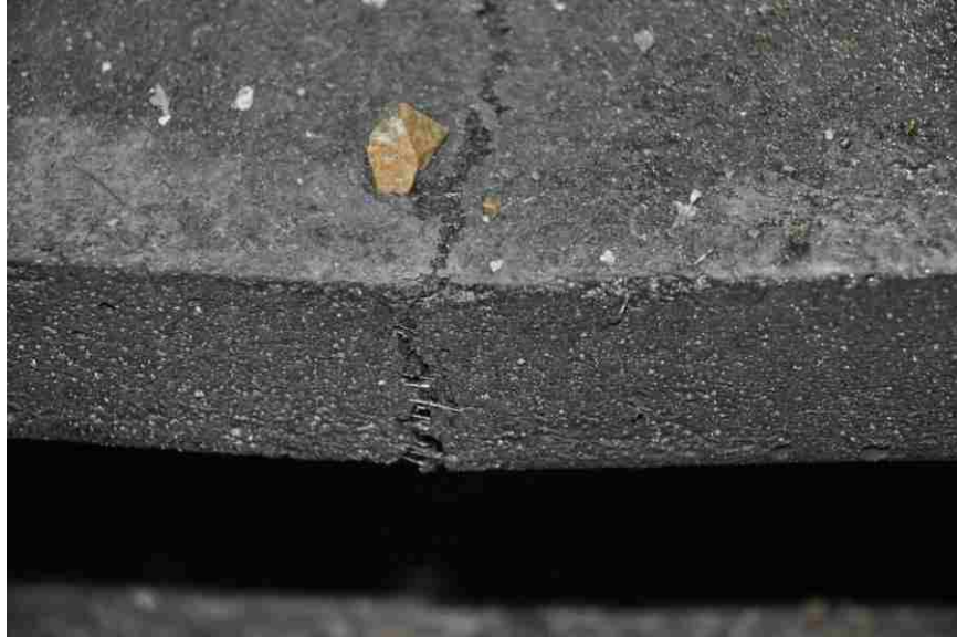
Figure 6.33. Crack development after detonation
