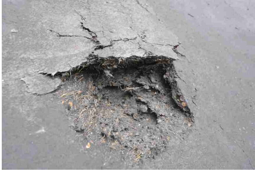
Figure 6.52. Close-up of spalling on H-3-6F-3.5
