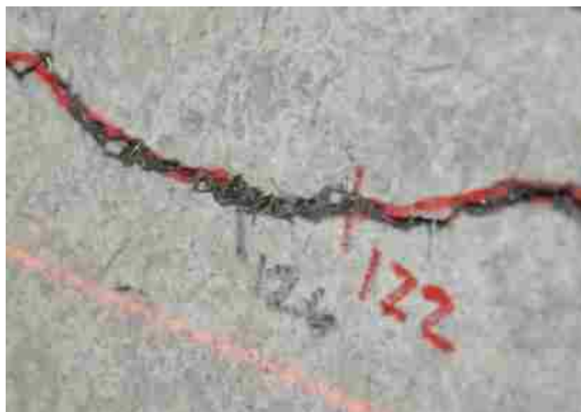
Figure 6.12. Fibers bridging bottom crack of I-2-6F-2
